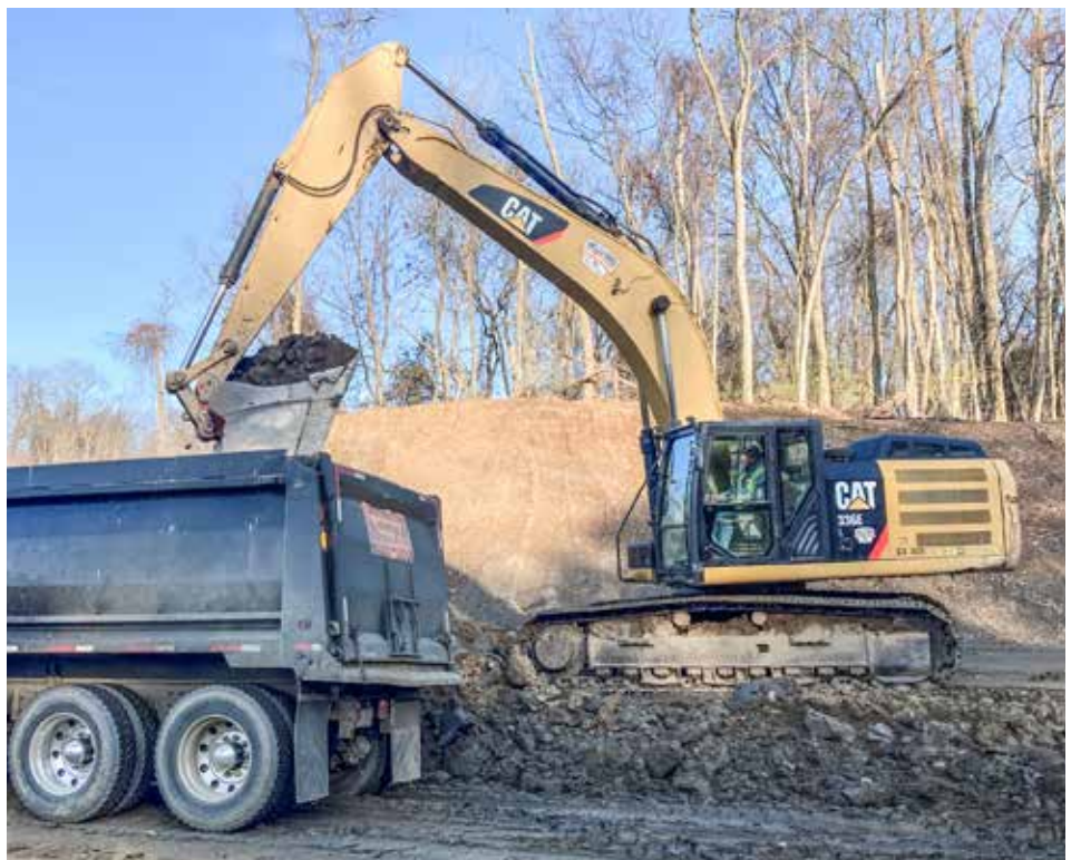
WORKING on the ramp project at S.R. 603 and U.S. Rt. 30 near Mifflin is Shelly & Sands.
