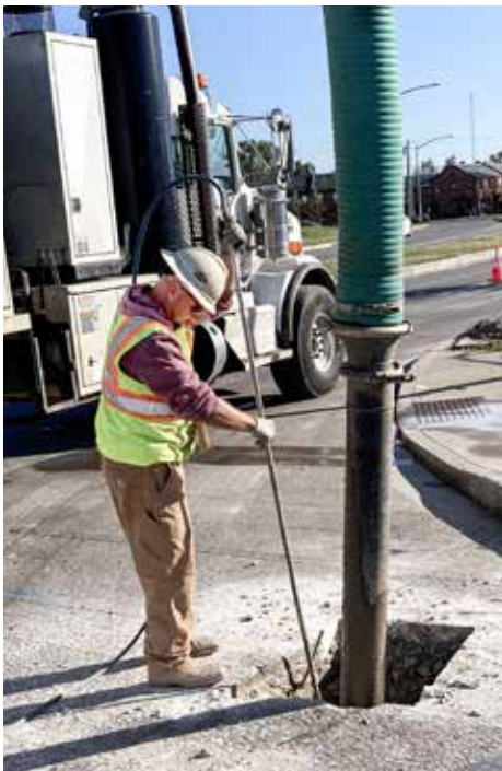
BUSY for Miller Pipeline in Dayton is Shaun McGill, operating a hydro excavator.
