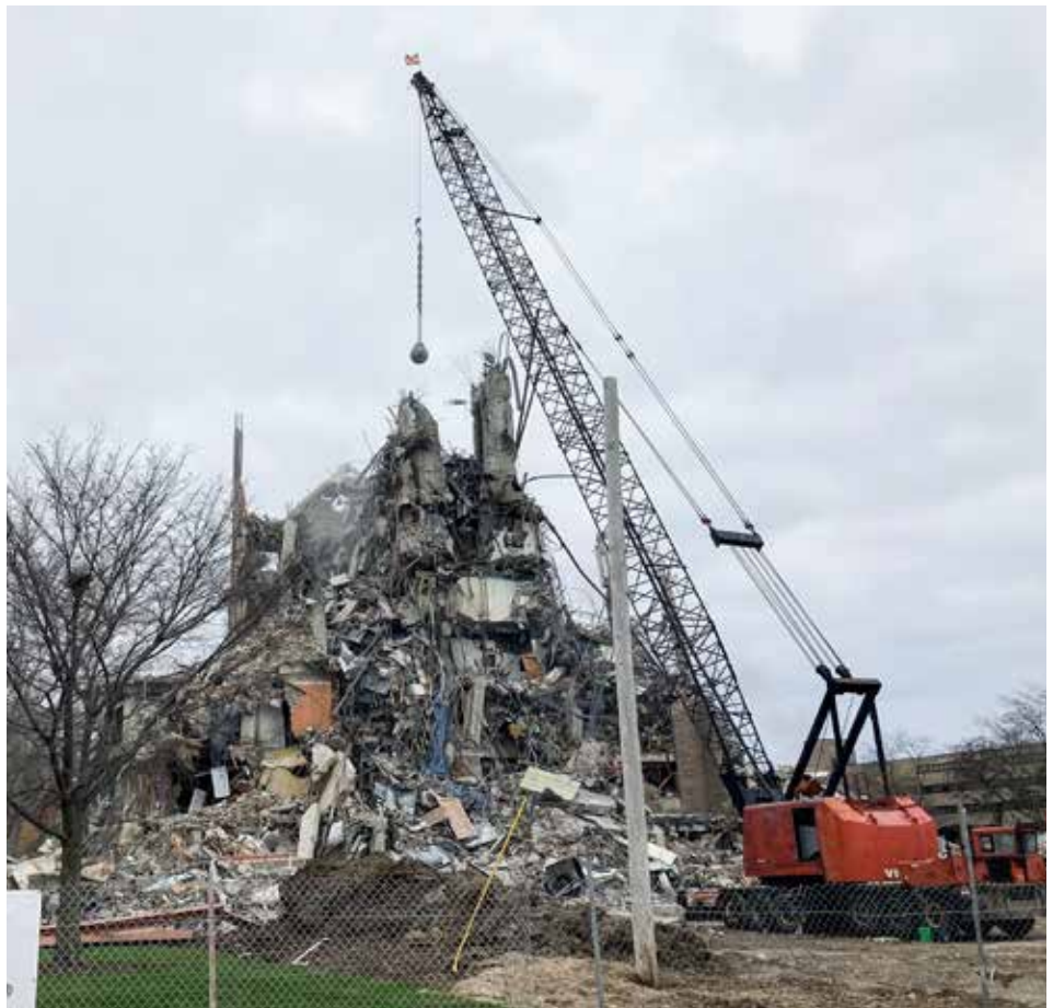
WORKING on a building demolition project in Bowling Green is Schaedler Enterprises.
