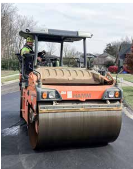
BUSY for Shelly Company, operating an asphalt roller in Springfield is Shawn Hanes.
