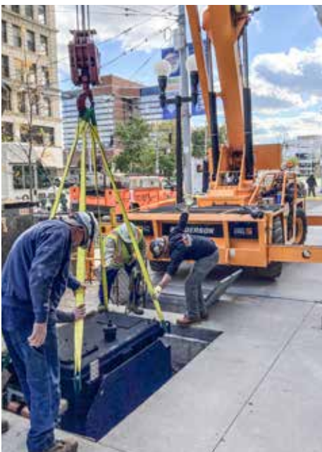
LOWERING an electrical transformer into an underground vault with a Broderson crane for PSC in Dayton is David Fisher.
