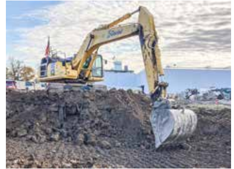
PERFORMING site work at Sandridge Food in Medina for Fabrizi Trucking & Paving is Dylon Bryant.
