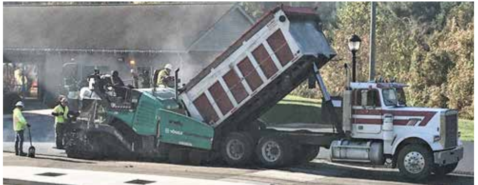
OPERATING a paver for Shelly Company at Southpoint Ohio in Lawrence County is Derrick Barnes .
