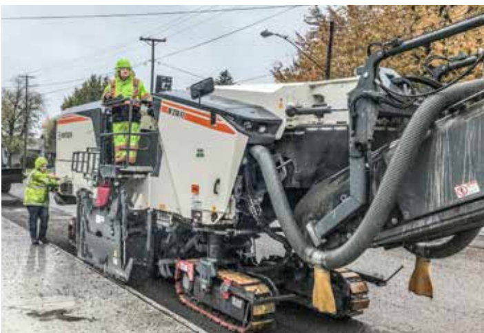
MILLING on S.R. 66 in Delphos for Ebony Construction Mike Johnson on the mill and Vaughn Keller in the broom.
