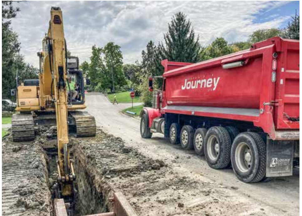
INSTALLING a water main for Kinnison Excavating in Centerville is Dave Kinnison, operating an excavator.
