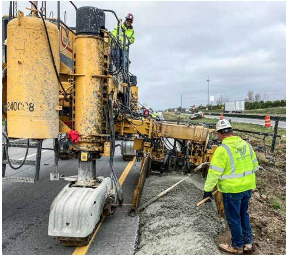
OPERATING a slip form concrete paver on I-70 In Springfield is Milton Dukas.
