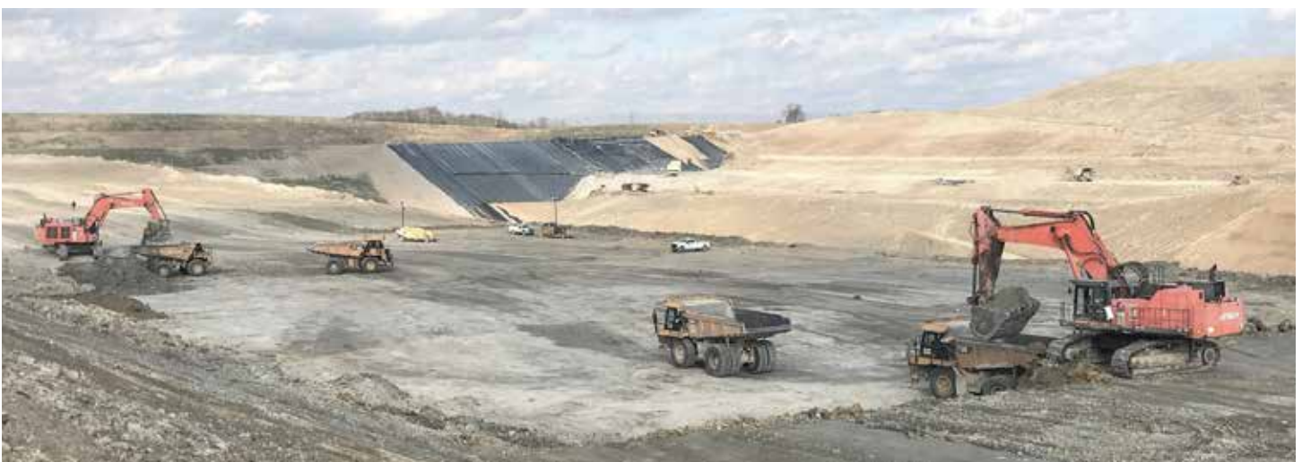
MOVING two million yards of dirt for a new cell at the Tunnel Hill Landfill in Perry County is Beaver Excavating.
