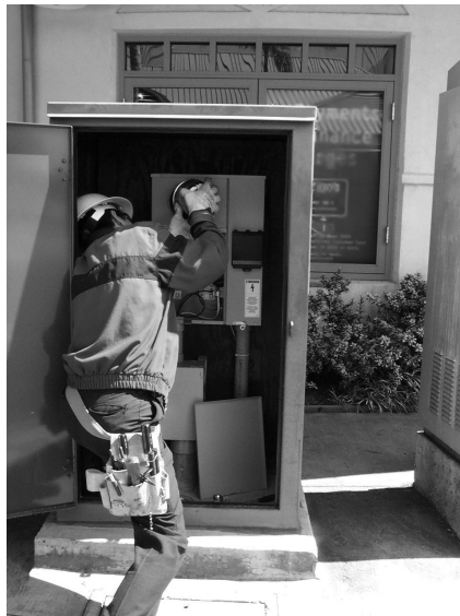
Figure 4-15. Freestanding meter enclosures shall have a minimum clearance of six inches between the top/sides of the meter socket and the lip of the enclosure opening to provide meter electricians with space to see and align meter blades with meter socket jaws.
