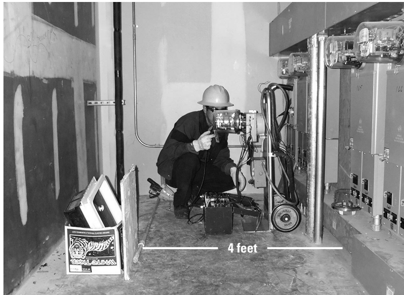
Figure 4-4. Meter Electrician performing a meter test. Notice the need for workspace clearance between the meter socket panel, and the pole on the floor.
